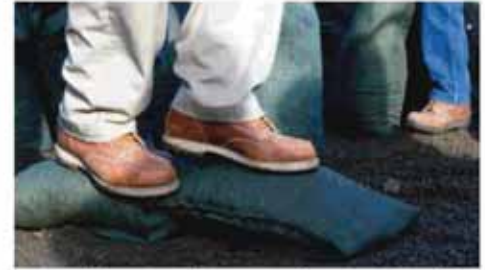
Place each succeeding bag tightly against and partially overlapping the previous one. Compact and shape each bag by walking on it.
